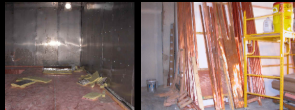
Silica Steel Mag Shielding and Copper RF Floor Shielding
