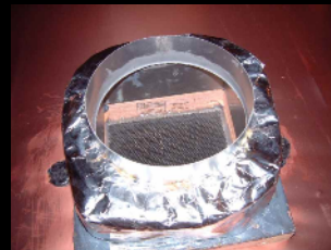
Duct with Baffle Filter
